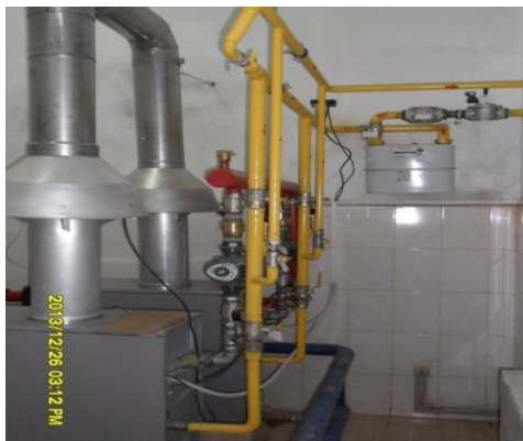
Boiler room (educational building No. 33, Lviv)
