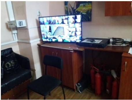
Security post of the main building (video surveillance, fire extinguishers, fire and security alarm panel)
