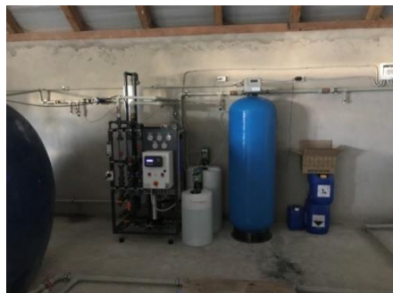
The water purification system of the Polytechnic-3 Recreational Camp
