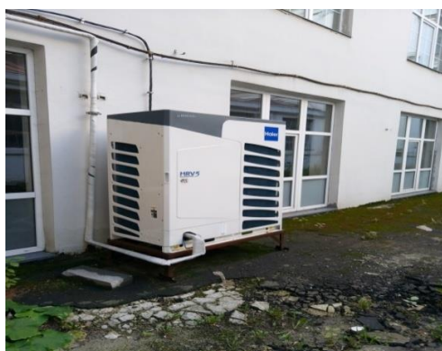
Heat pump with recuperator (main building, Lviv)
