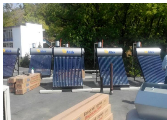
Solar helio system (dining room, the Polytechnic-2 Recreational Camp, Ukraine)
