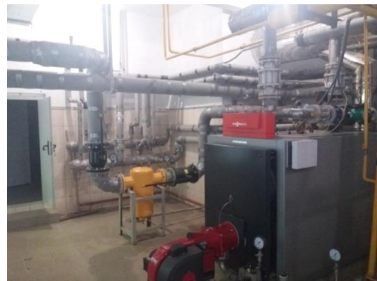
Boiler room (educational building No. 21, Lviv)
