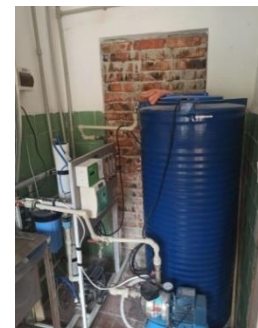
The water purification system of building No. 1 of the Polytechnic-2 Recreational Camp
