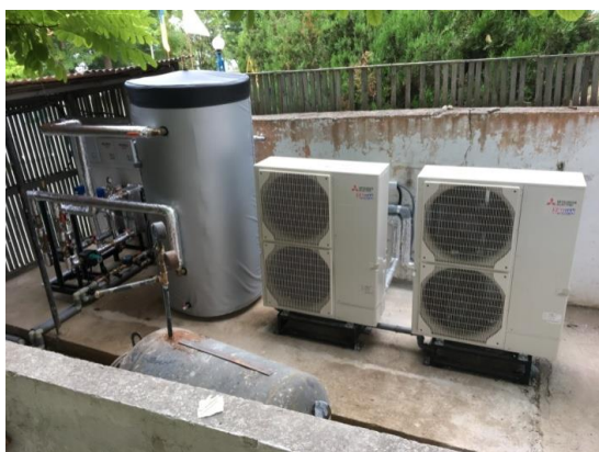
The heat pump (dining room, the Polytechnic-2 Recreational Camp, Ukraine)
