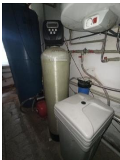
The water purification system of building No. 4 of the Polytechnic-2 Recreational Camp
