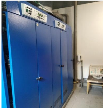
Boiler room (educational building No. 7, Lviv)
